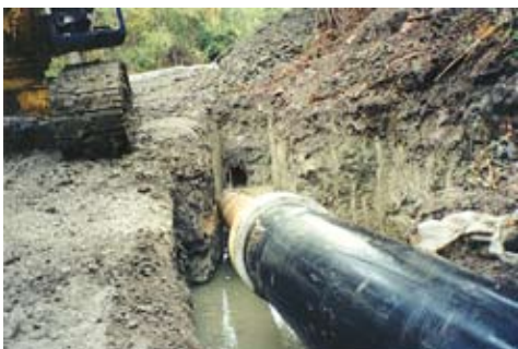
Rehabilitation of Hillsborough’s mini basins and trunk sewer involved pipe bursting, fold-and-form, and conventional pipeline replacement methods.
