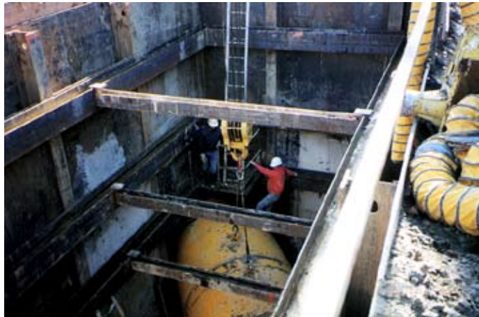
Los Angeles County's Trunk Relief Interceptor project required significant tunneling beneath city streets.
