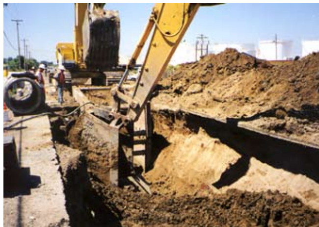
Stockton’s Westside Sewer Interceptor alignment crosses developed urban areas, underdeveloped farmland with some peat deposits, a river, a deep water channel, and a military facility.
