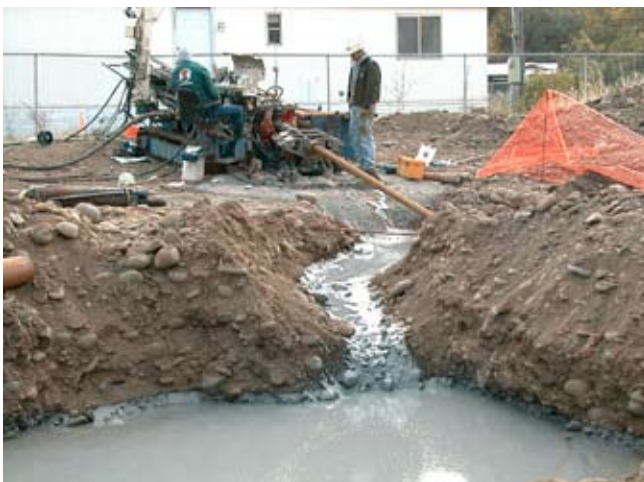
A sub-river crossing using horizontal directional drilling proved to be the most cost-effective and environmentally-friendly construction alternative for replacement of Shady Cove's Lift Station No. 2 force main.
