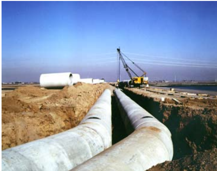
Carollo provided routing, design, and construction services for Phoenix's Southern Avenue Interceptor.
