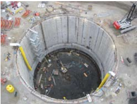
Currently under construction, Portland's Swan Island Pump Station is believed to be one of the deepest of its kind in the world.
