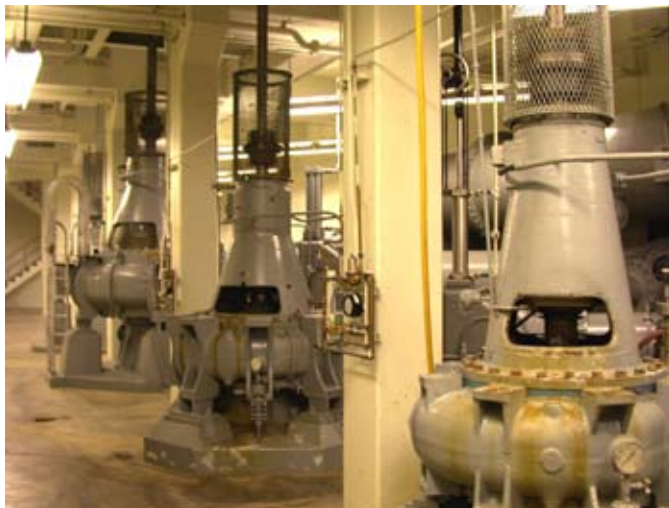
Carollo provided a comprehensive program for future design and operational changes and designed a capacity upgrade of King County's Matthews Park Pump Station.
