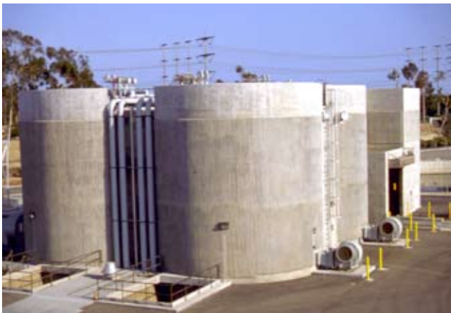
Orange County's biosolids handling facility combines state-of-the-art pumping, storage, and loading technology with computer automation in a system capable of transporting nearly 600 cy of biosolids cake daily.
