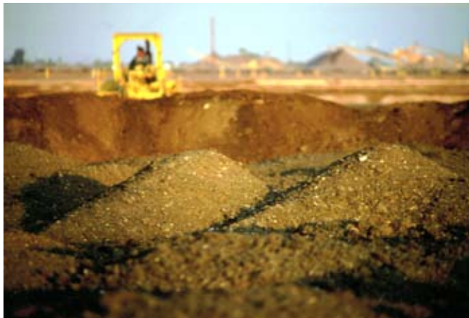
Sludge dewatering options investigated as part the Phoenix Residuals Management Facilities Plan included mechanical methods, solar dewatering, thermal drying and composting.
