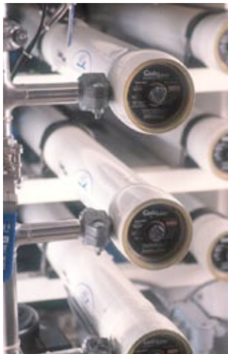
Carollo evaluated installation of RO treatment, as shown.
