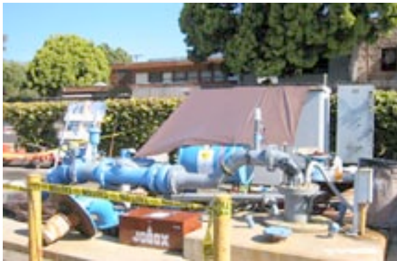
Corporation Yard Well located at the City of Santa Barbara yard.
