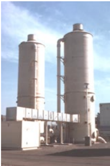
Carollo designed a 6,000-gpm air stripping facility at the Newmark site in San Bernardino, California.
