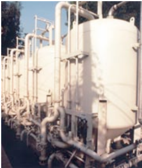
Carollo designed a groundwater remediation program for the 17th and Sierra Street Wells.
