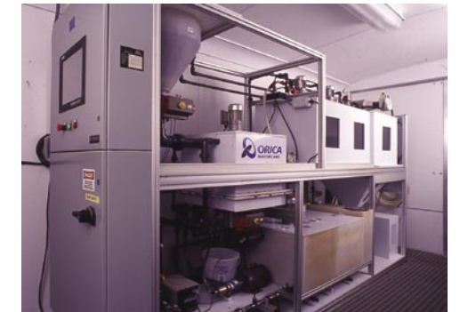
MIEX ® process pilot plant.
