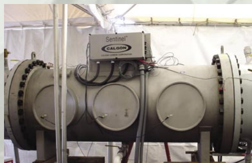
Validation of the Calgon 36" reactor.
