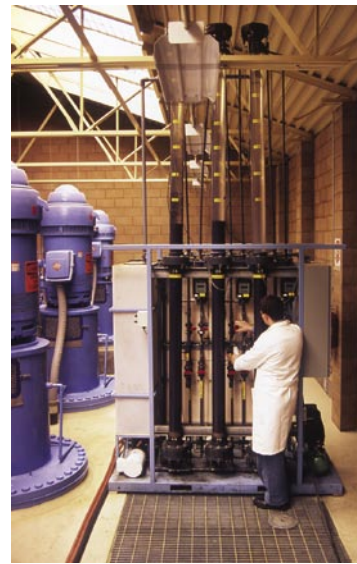
Pilot GAC columns at Palmdale.
