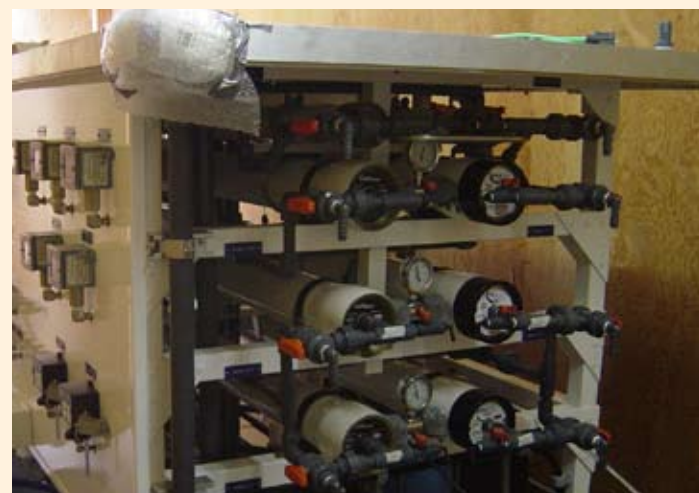
A dendrimer anti-scalant was added to the feedwater of the pilot-scale RO membranes to evaluate the improvement in system recovery.
