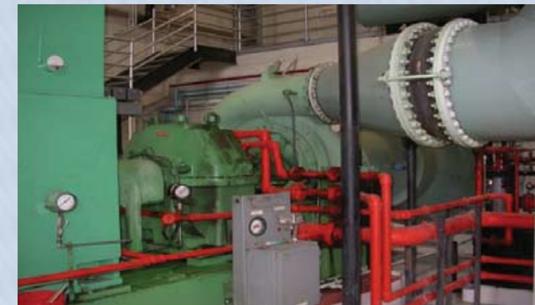
Understanding the tariff impacts and coordinating large equipment starts can save significant money.
