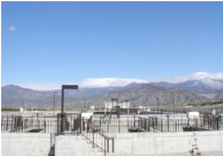
Carollo evaluated perchlorate treatment technologies as part of a water feasibility investigation.
