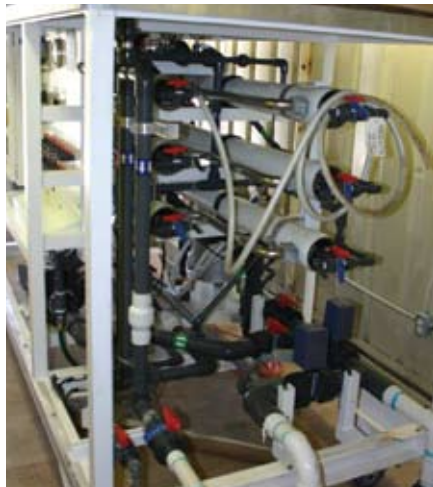
Multiple RO recoveries and treatment options will be evaluated.
