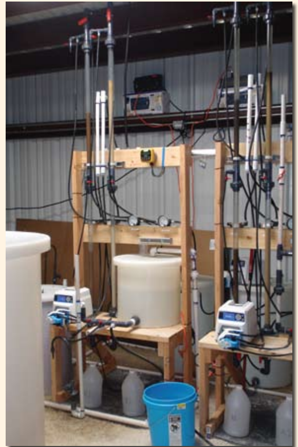
Carollo used these small-scale column skids for single-use media testing during the pilot study for the City of San Angelo, TX.
