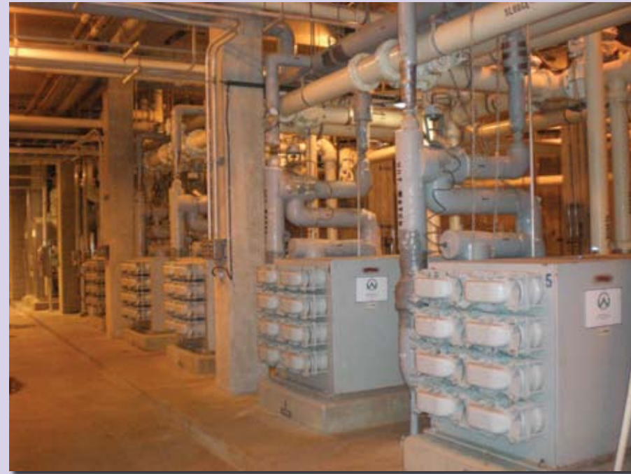
Dallas Water Utilities detected scaling in sludge heating and recirculation piping and heat exchangers at their Southside Wastewater Treatment Plant. Carollo's study of scale formation and mitigation led to the development of a thermal imaging technique for monitoring scaling in heated sludge piping.
