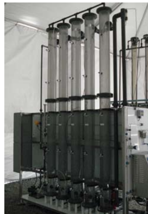
Ozone pilot skid at Contra Costa Water District, CA.
