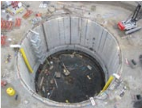
Currently under construction, Portland's Swan Island Pump Station is believed to be one of the deepest of its kind in the world.
