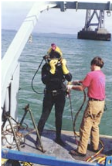
Carollo coordinated and led team efforts during the 1995 and 1996 repairs to both Outfalls No. 1 and No. 2.
