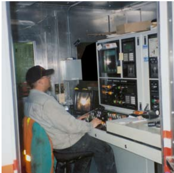
A state-of-the-art control console, located in a portable container, allowed operators to remotely control the electronically-powered MTBM.
