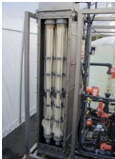
MBR efficacy testing at King County's Hollywood Pump Station helped determine the feasibility of treating wastewater to a level suitable for agricultural irrigation.
