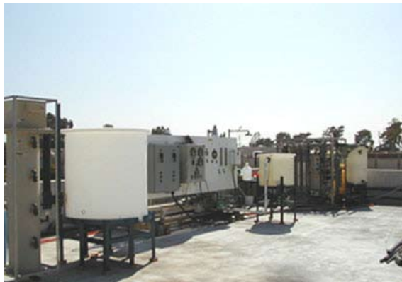
IMANS® was technically proven during an 18-month pilot test at the Orange County Sanitation District.
