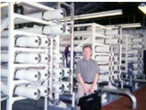
Carollo is providing engineering services for the expansion of the SIPSD's RO treatment plant from 1.5 to 3 mgd.
