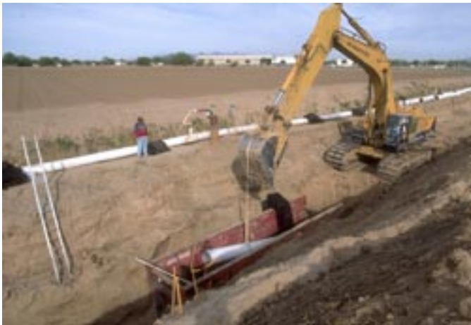
Carollo has assisted El Paso Water Utilities with planning, design, and construction of some of the area's largest potable water delivery systems.
