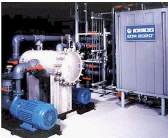
The new EDR facility was started up in 1996 with excellent results.
