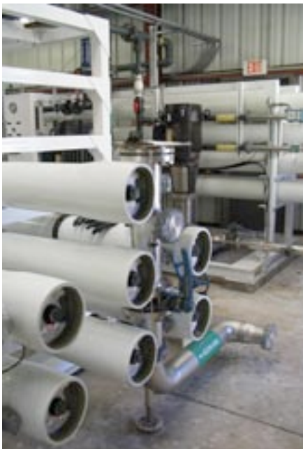
Carollo provided engineering services for the design/build expansion of the Golden Gate RO Water Treatment Plant.
