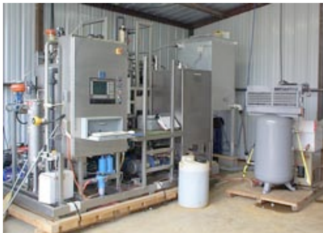
Coagulation/microfiltration was one of five arsenic treatment technologies evaluated for the City of Chandler over an 8-month period.
