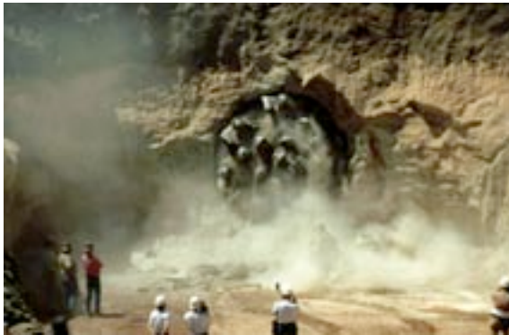
The team managed 20 individual construction contracts including four miles of 12-foot-diameter tunnel bored through the River Mountains.
