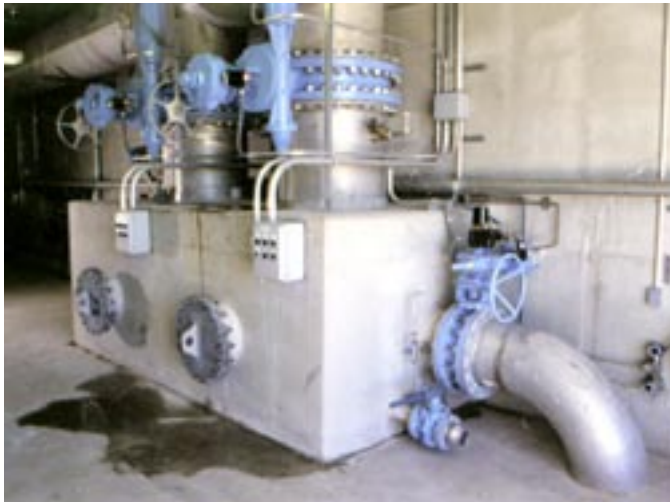
The high-rate BAC filters at the Appleton Water Treatment Facility remove 1.5-2.0 mg/L of BDOC at a 20-minute EBCT.
