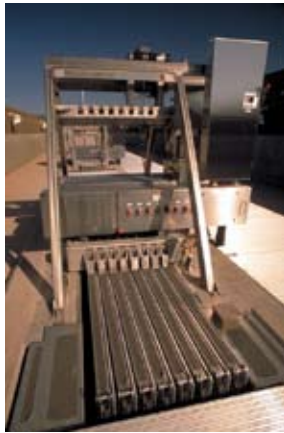
Carollo designed one of the largest UV disinfection systems in the state of Arizona at the Cave Creek Water Reclamation Plant.
