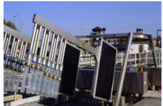
The Vallejo Sanitation and Flood Control District uses UV disinfection accommodate flows up to 30 mgd.
