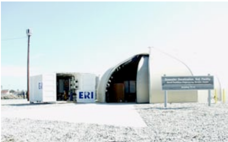
The ADC facility will demonstrate Pacific Ocean desalination at energy consumption rates three times lower than thought possible.
