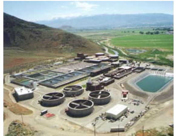
Carollo is assisting with NPDES permitting planning and design for the expansion of the Truckee Meadows Water Reclamation Facility.
