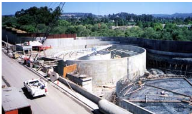
The proximity of the Santa Cruz Wastewater Treatment Plant to protected wetlands and the Monterey Bay Marine Sanctuary presented some special challenges to Carollo’s construction management effort.
