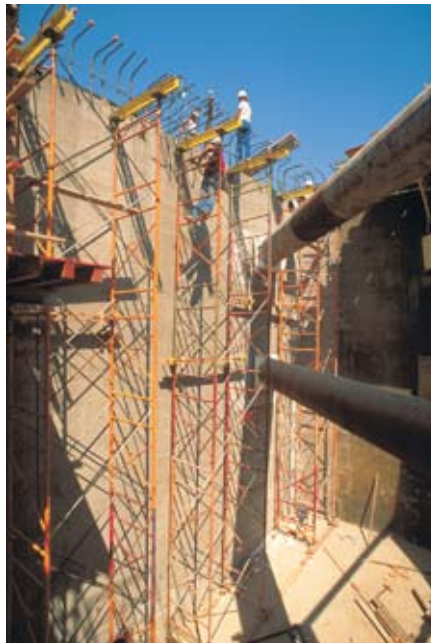
Construction of EBMUD’s wet weather storage basin required a state-of-the-art shoring system for the deep excavation in bay mud.
