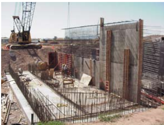
The Greenway Water Treatment Plant was designed for conventional treatment in combination with ozonation and biologically active filtration.
