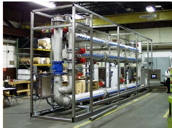
To meet water quality objectives, the upgrade of the Brazos River Authority Water Treatment Plant included new low-pressure membranes and reverse osmosis.
