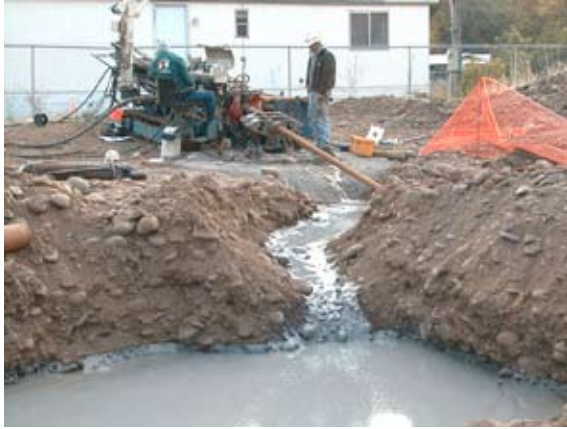
A sub-river crossing using horizontal directional drilling proved to be the most cost-effective and environmentally-friendly construction alternative.
