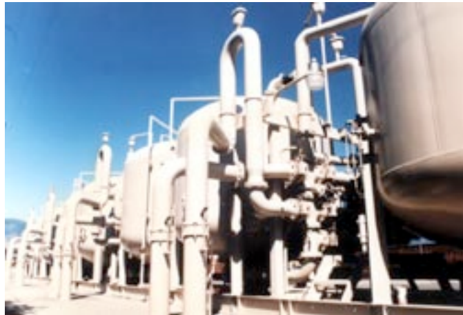
Carollo selected granular activated carbon to treat groundwater contamination in potable water supply wells.
