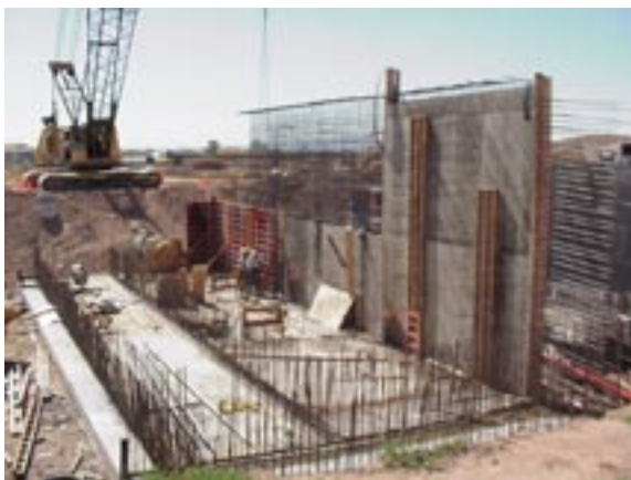
The Greenway Water Treatment Plant will meet Peoria's water needs by 2002.
