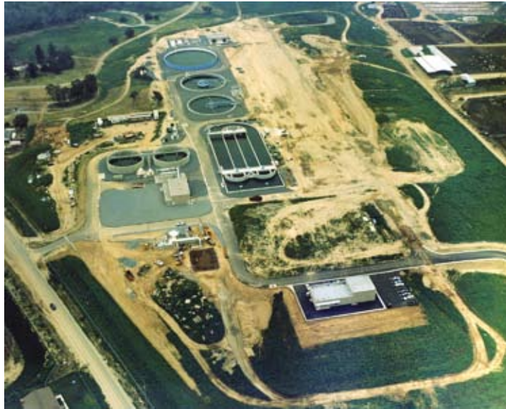
A partnering approach helped to maintain excellent communication with all stakeholders during construction of Western Riverside County's Regional Wastewater Treatment Facility.
