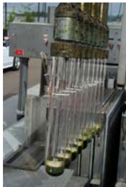
Carollo has tested and validated UV lamps and sleeve cleaning technologies.
